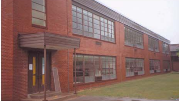
BEFORE... aging school windows are high maintenance, inefficient and undesirable.
